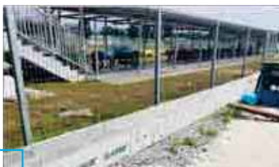
Picture: MRT 2 - Cable Troughs
