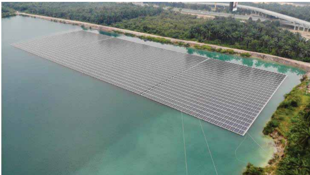
Picture: 9.9MWp DC floating solar plant in Dengkil, Selangor
