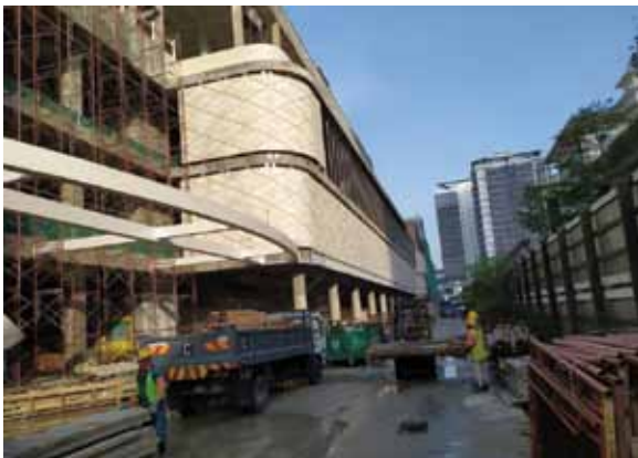
Picture: Bukit Jalil Pavilion 2 Shopping Mall – Façade walls constructed using UHPC that are highly customised, curved with three pattern features, pre-finish with everlasting pigmented homogeneous colours. Large and lightweight panels allow quick and fast track construction.
