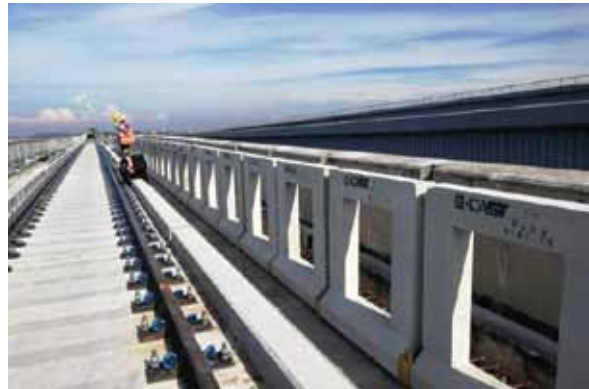
Picture: MRT 2 Cable Trough & Walkway
