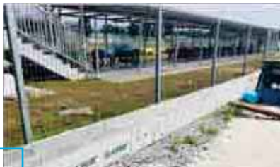
Picture: MRT 2 - Cable Troughs
