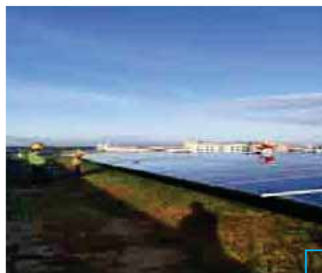
Picture: 58.8MWp DC capacity solar plant in Kuala Kertih, Terengganu
